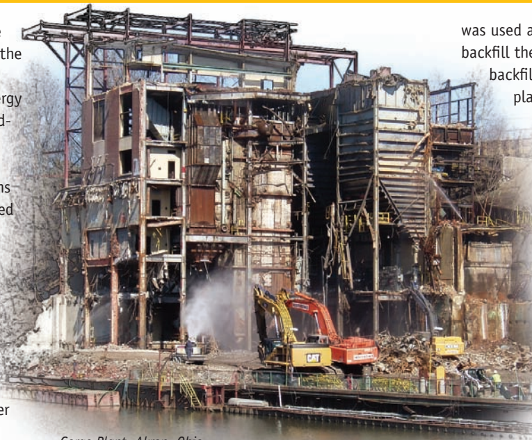
Gorge Plant, Akron, Ohio
