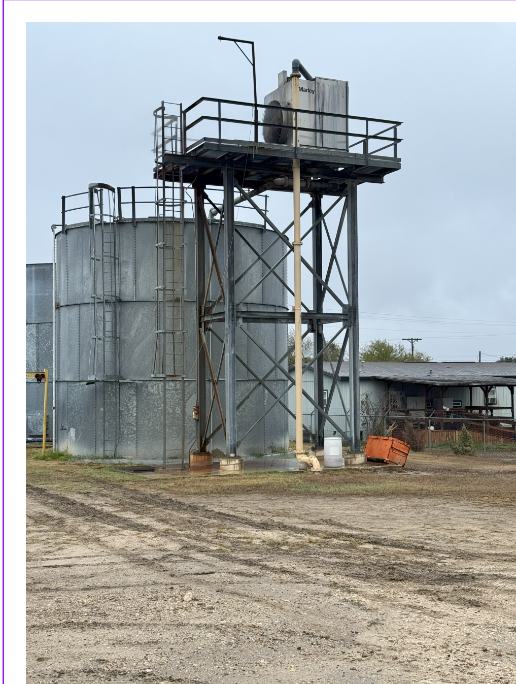
LEFT: Water Plant Cooling Tower Structure is failing and needs immediate repair.
