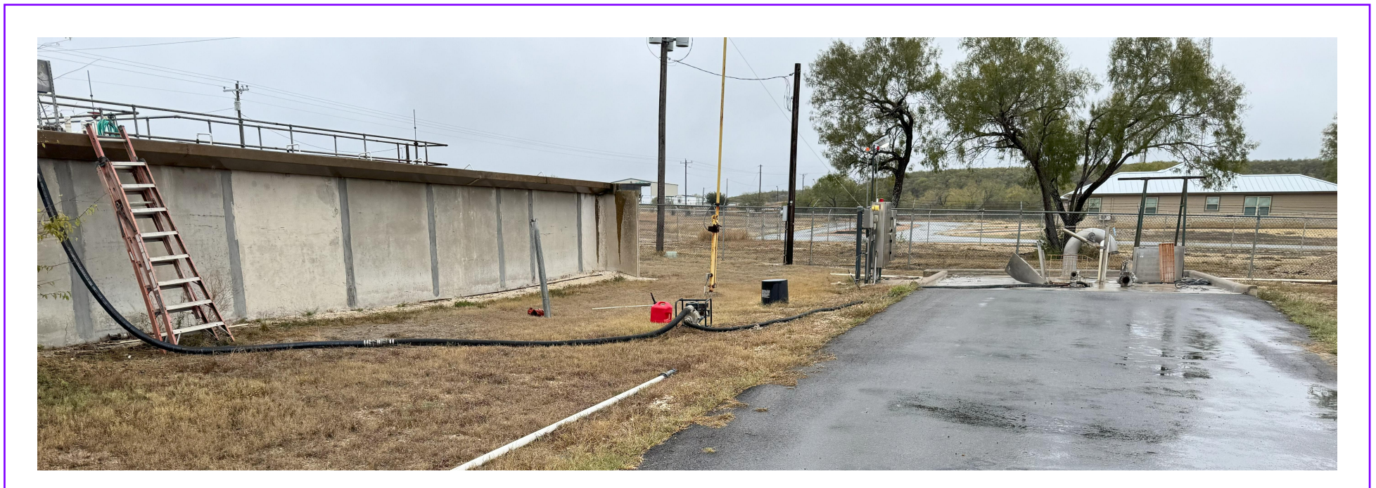
BELOW: The Influent Lift Station Pumps at the Wastewater Treatment Plant have failed and need to be replaced.
