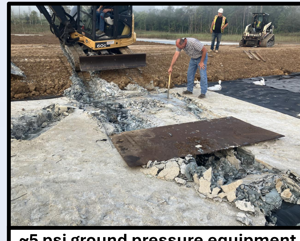
~5 psi ground pressure equipment sinking directly into the CCR surface
