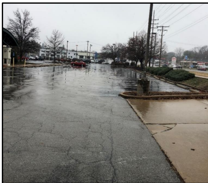
Pic 1.1: Looking west at east entrance with minor cracking observed
